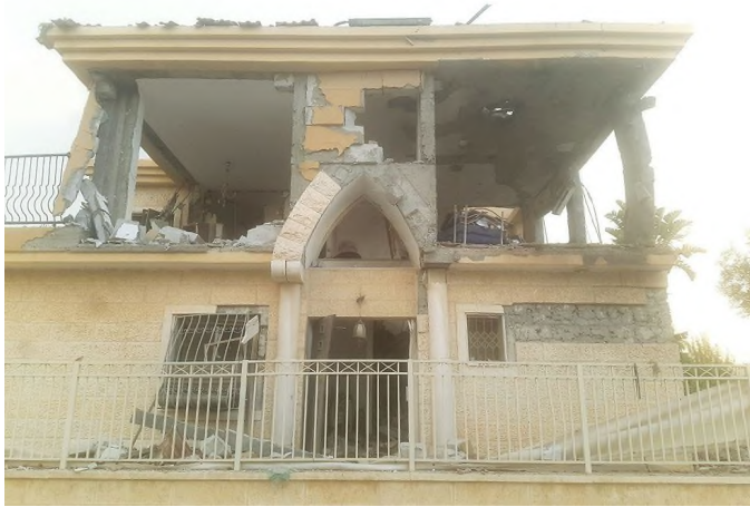
The house that suffered the direct rocket hit
